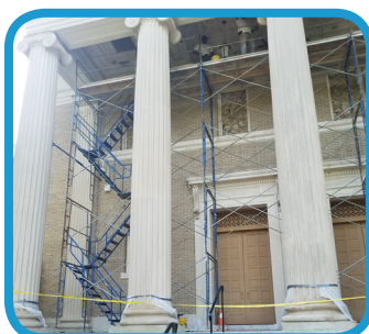
To repair the soffit, a metal work scaffold was erected, including a temporary access stair.
