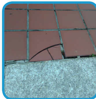
Over time, standing water and freeze-thaw cycles had cracked landing pavers and deteriorated mortar joints.
