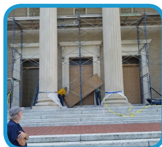
Poorly fitting and worn exterior sliding doors were removed to access the hidden support hardware.
