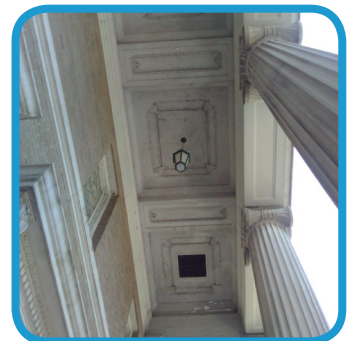
The three-story high plaster soffit had begun to crack and shed its paint finish.
