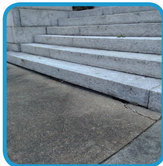
The gap between the concrete walk and the stone stair riser had become a tripping hazard.
