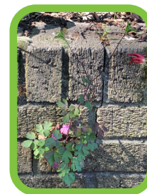
A native columbine grows in the wall.
